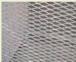
▼ Deteriorated polyester coating after 6 years.
