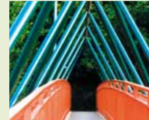
◀◀ Plascoat PPA 571 in good condition after 18 years.
